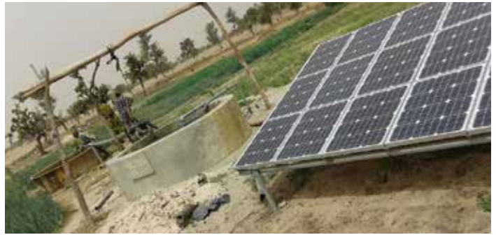
Image 1: Solar system for wells in Gossas
