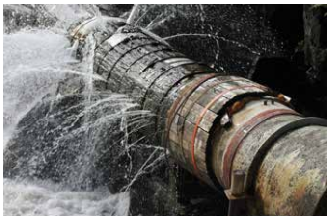
Image 9: Aging water infrastructure
